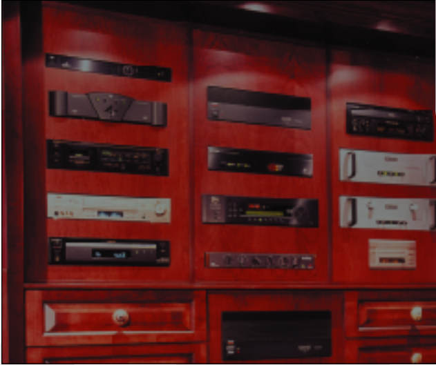
Installation by Connected Technologies, Colorado Springs, CO
