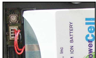
Battery Cable Plugged In
