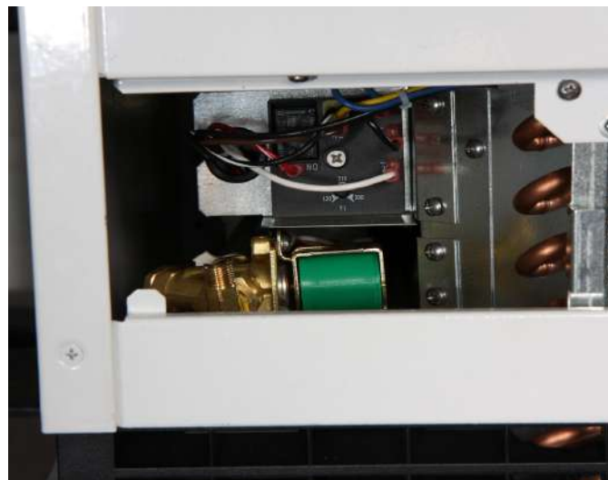
Inlet Water Solenoid Valve
