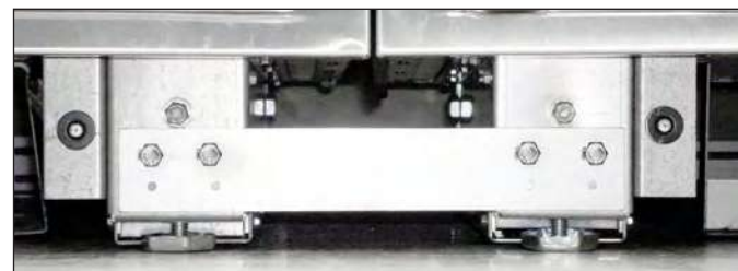
FIG. 18. Installed joining bracket.
