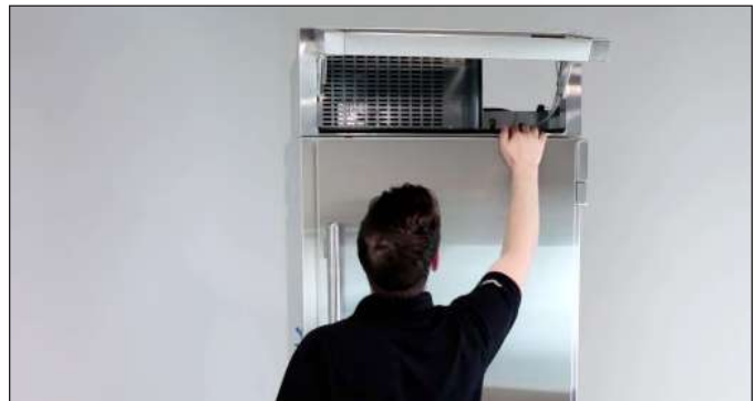
FIG. 3. Be sure to inspect the rainshield.
