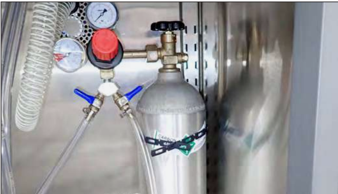
FIG. 9. Always strap the CO 2 cylinder into the appliance.
