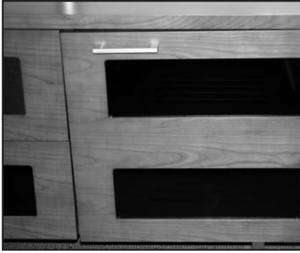
INCORRECT! Door is out of alignment with the rest of the unit.
